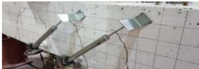
(c) Post-cracking stage
