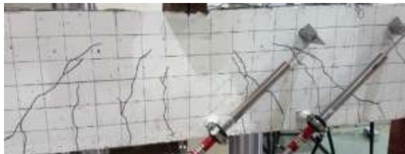
(c) Post-cracking stage
