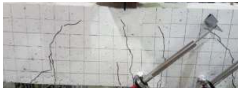
(c) Post-cracking stage
