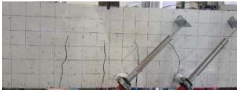
(c) Post-cracking stage
