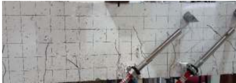
(c) Post-cracking stage
