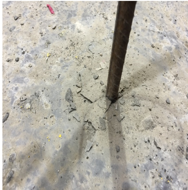
Figure 30: Crushing and cracking of concrete surrounding the rebar at the surface
