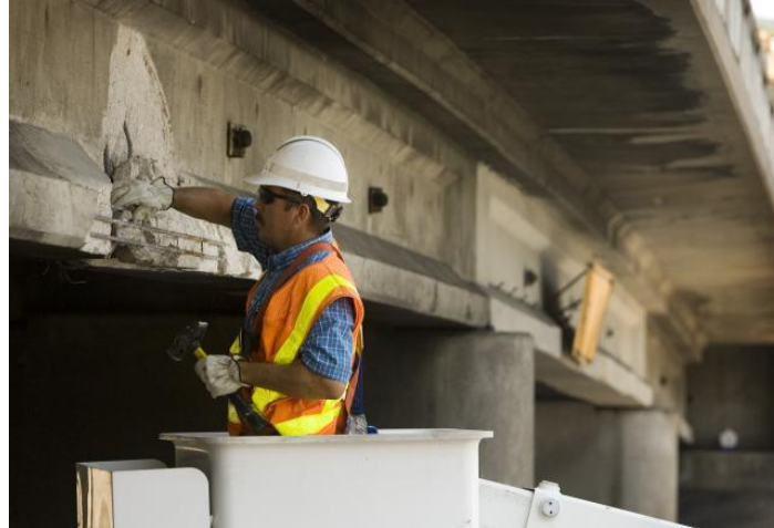
Fig. 1.2: Typical damage in a prestressed concrete girder due to over-height truck impact [2]
