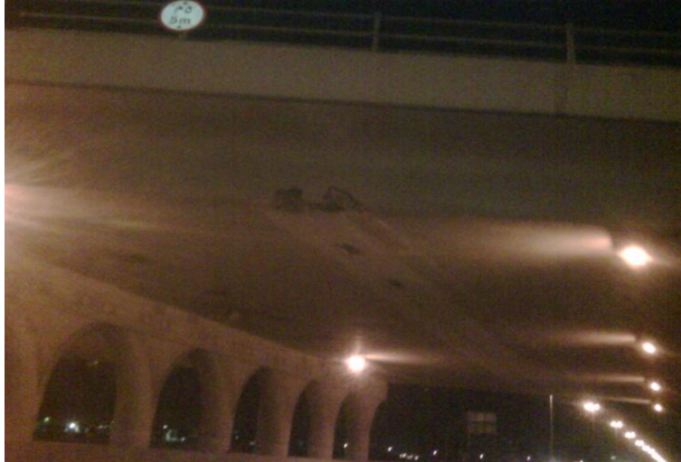
Fig. 1.3: Example of minor damage of a bridge in UAE (photo taken by author)
